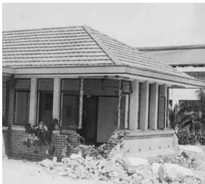
Women's Rest after the Hawke's Bay earthquake on 3 February 1931 from the Tennyson Street side of Memorial Square. The building was badly damaged by the earthquake. Photographer probably Frank L. Moodie, architect. Source: MTG Hawke's Bay objects nos. m90/31, 7256 m, 6620
